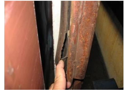
Bad seals can cause leaks
